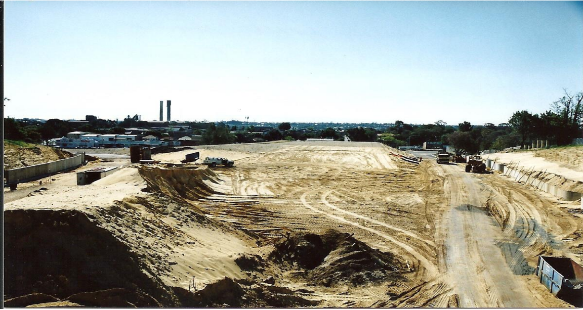
Taken from the new pedestrian bridge looking towards Great Eastern Highway showing the overpass bridge abutments starting to take shape.
