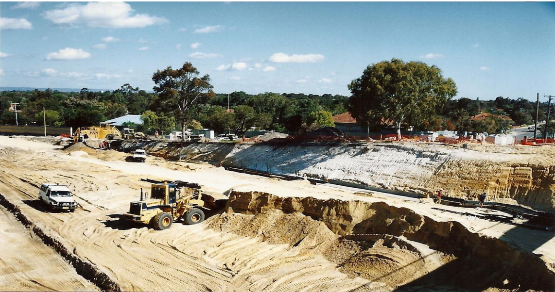
Taken from the pedestrian bridge showing the depth of the cutting. Gallipoli Street can be seen on the right.
