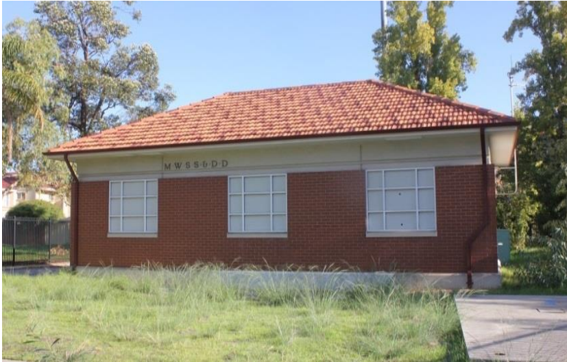
The Sewerage Depot At Western End Of Hordern St Victoria Park – As it is Today - (May 2023)
